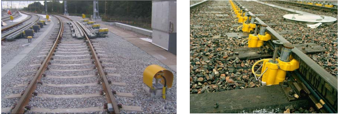
Figure 48. The new track brake system at Hallsberg marshalling yard before the snow fall 41 .
