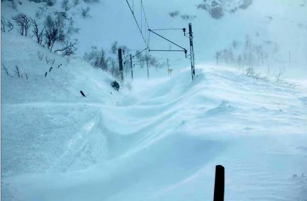
Figure 40. The line close to the place for the accident covered with snowdrift the day after the accident. 31
