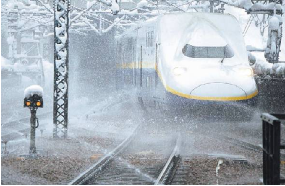
Figure 47. A Japanese water sprinkler system in practice on East Japan Railway Company. Notice the amount of snow on the catenary and the ground free from snow 39 .
