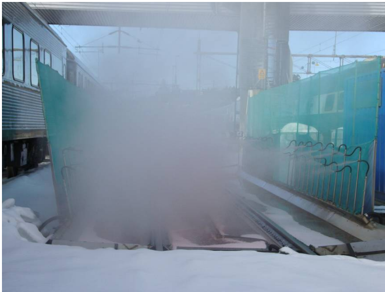
Figure 33. The propylene glycol de-icing at Hagalund demonstrated in 2010 without any vehicle. It can be seen that a fairly low pressure is used for the de-icing. The nozzles are located both on the sides and in the middle between the tracks.
