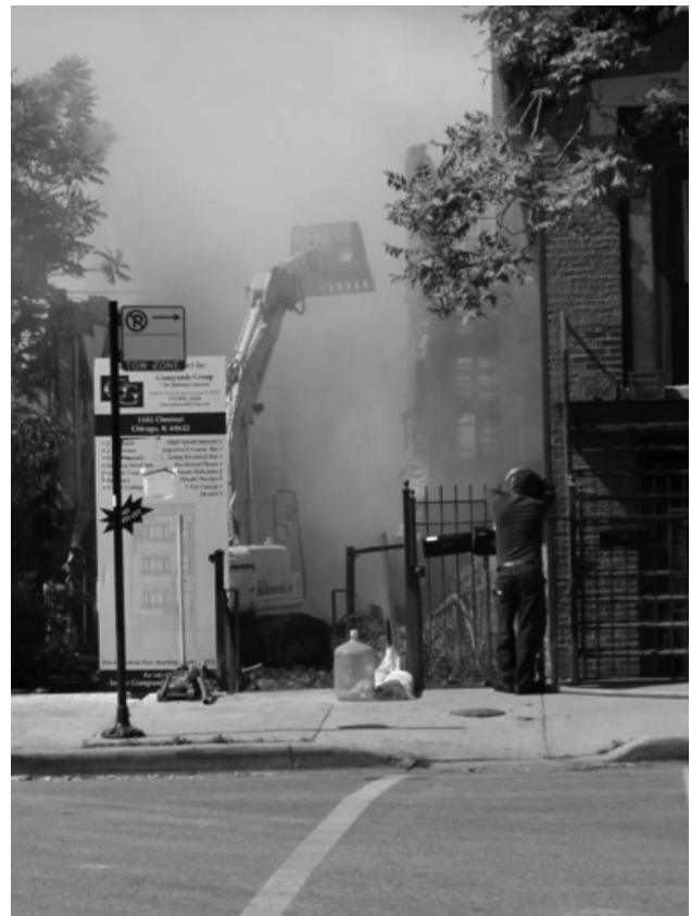
Photo 3. No dust suppression used at a demolition site in Chicago. Source: University of Illinois at Chicago
