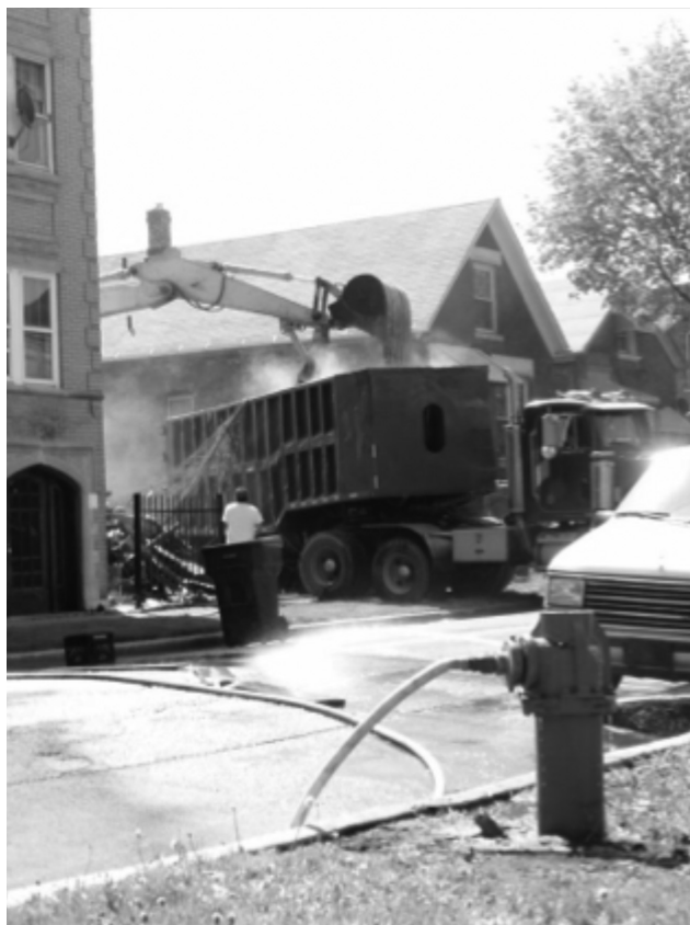
Photo 4. Limited dust suppression in use at a Chicago demolition site. Source: University of Illinois at Chicago
