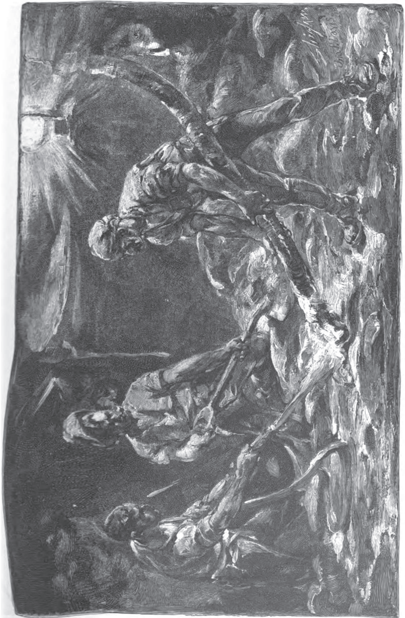
At Work in a Pneumatic Caisson—Fifty feet below the Surface of the Water.
